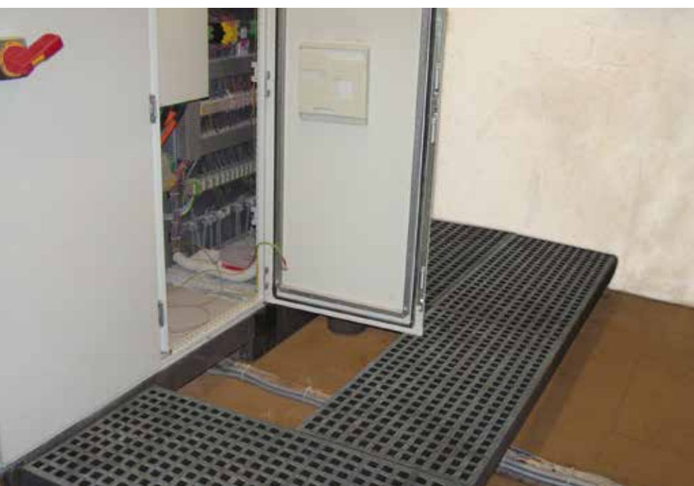
Non-conducting double floor
